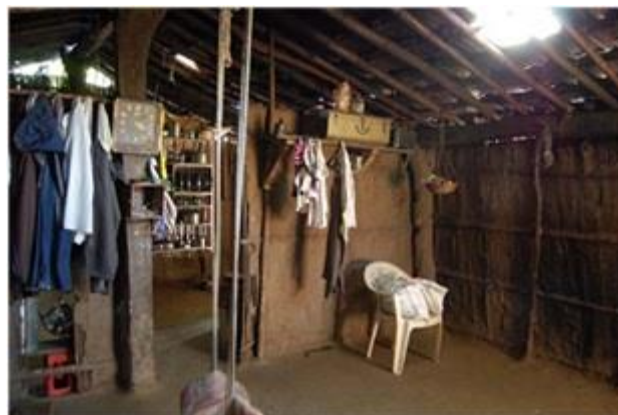
Photo 8: Timber pillars and beams, bamboo purlins, hay and hemp used as walls.
