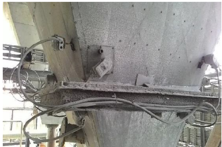
Figure 3, Heating coils location
