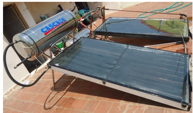
Fig. 4.1. Photograph of new set of series system taken at Tiruchirappalli, Tamilnadu, India, (longitude 78°43', latitude 10°46').
