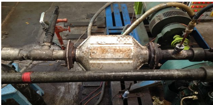
Fig.2.2. Photographic view of SCR
