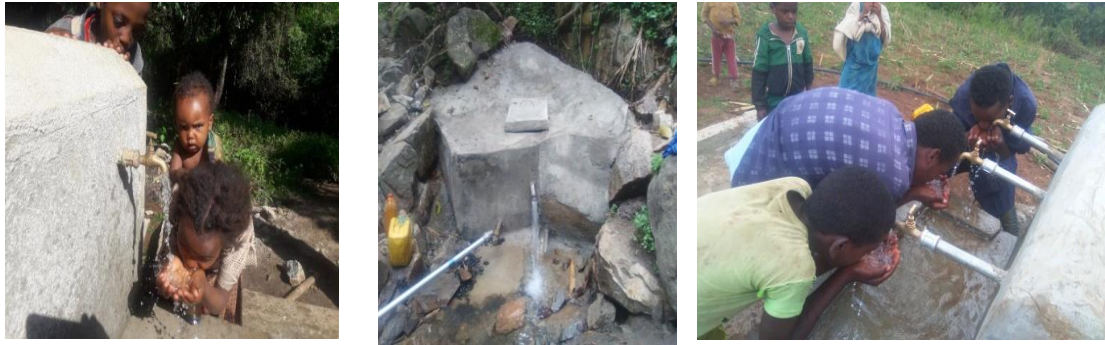
Figure 5: Spring capped structure and Community water points.
