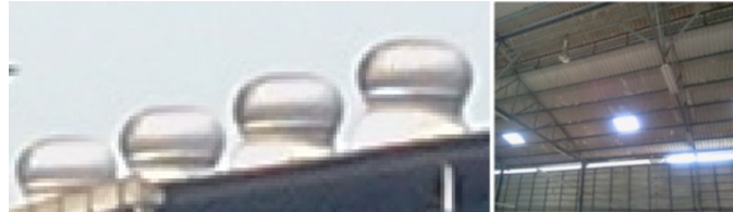
Fig. 1 Existing rooftop ventilators in Thailand (factory rooftops)
