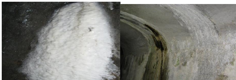
Fig. 1 White Leachate deposit in the Power House Complex Fig. 2 White, Black and Brown Leachate deposit in Dam Gallery
