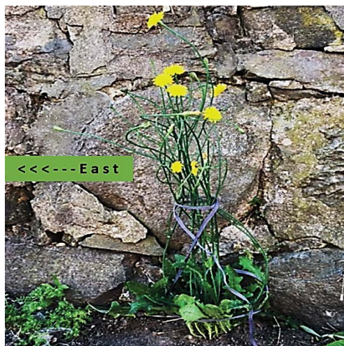
Figure 1b. 24-inch tall (0.6 meter), 12-stem Hypochaeris radicata catsear plant, having penetrated an asphalt-macadam sidewalk. The vertical lift capability of plant estimated at a remarkable 70-lbf (32 Kg). The flowers demonstrate the “positive phototropic effect”.
